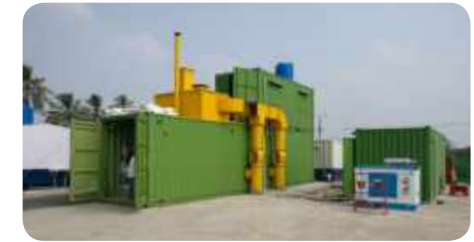
Faecal Sludge Treatment Plants
