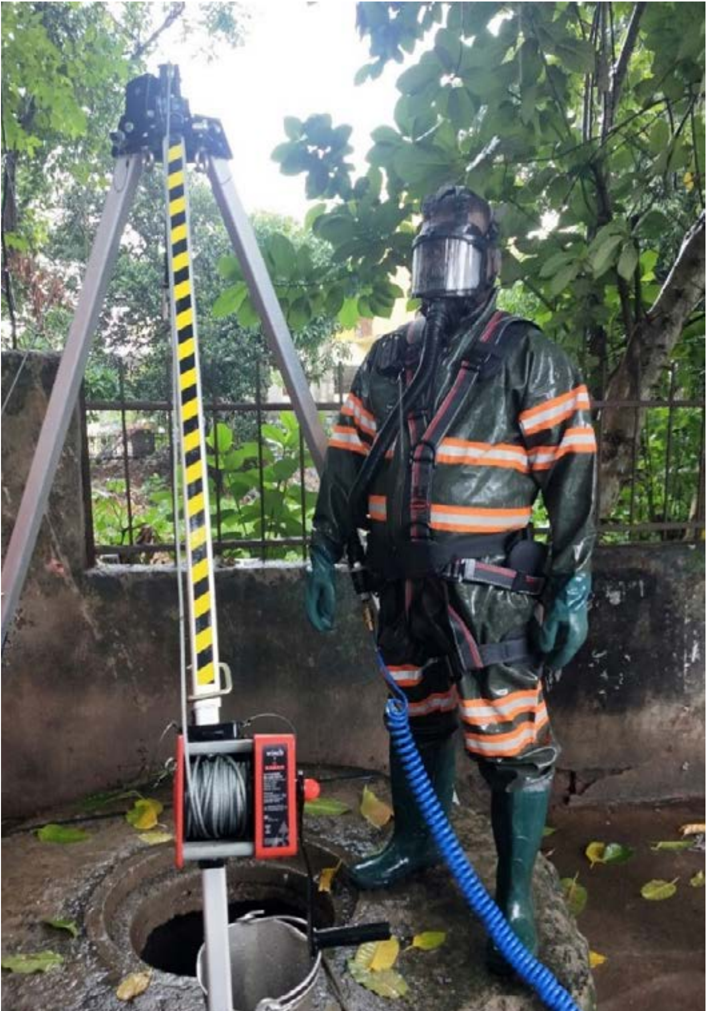
A Sewer Entry Professional (SEP) engaged in manual cleaning of a sewer line
