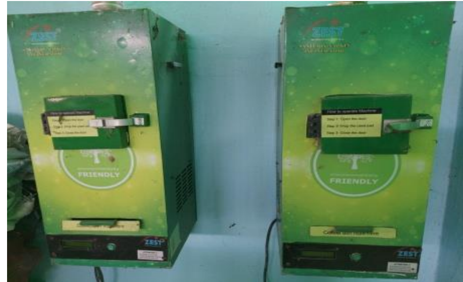
Incinerators for Sanitary waste disposal
