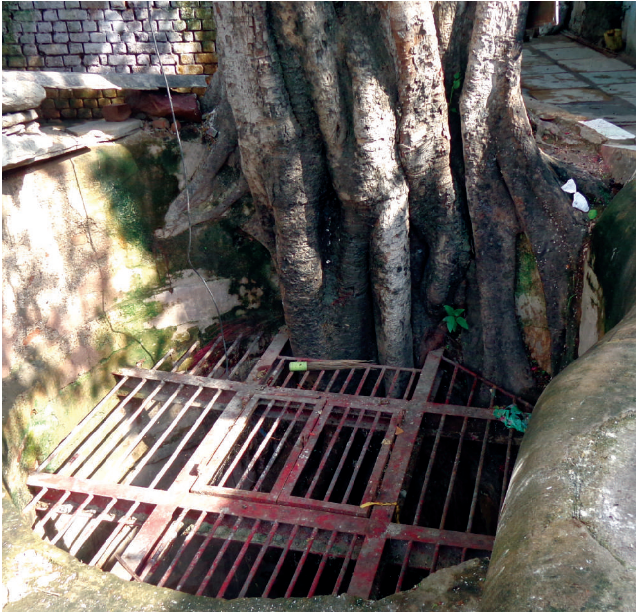
Vegetation is damaging the structure
