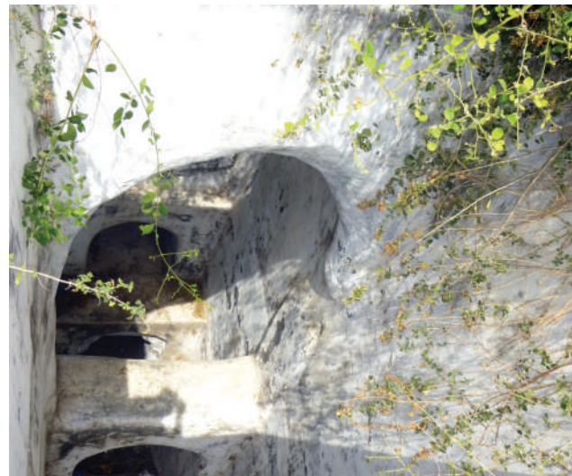
The arches have lost their original character
