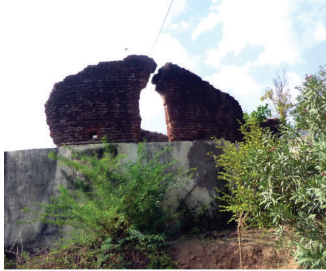
Part of well extends above ground
