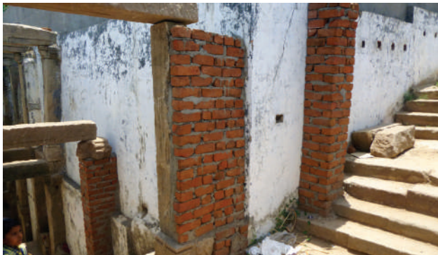
Improper materials have been used for restoration
