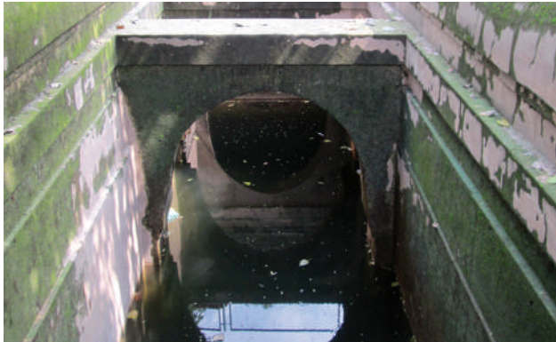
Dirty water accumulates in the well
