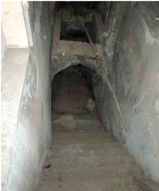
The inside of the well is dirty and degraded
