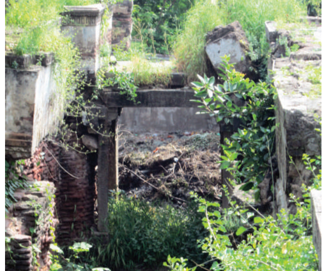
The well has been covered by vegetation
