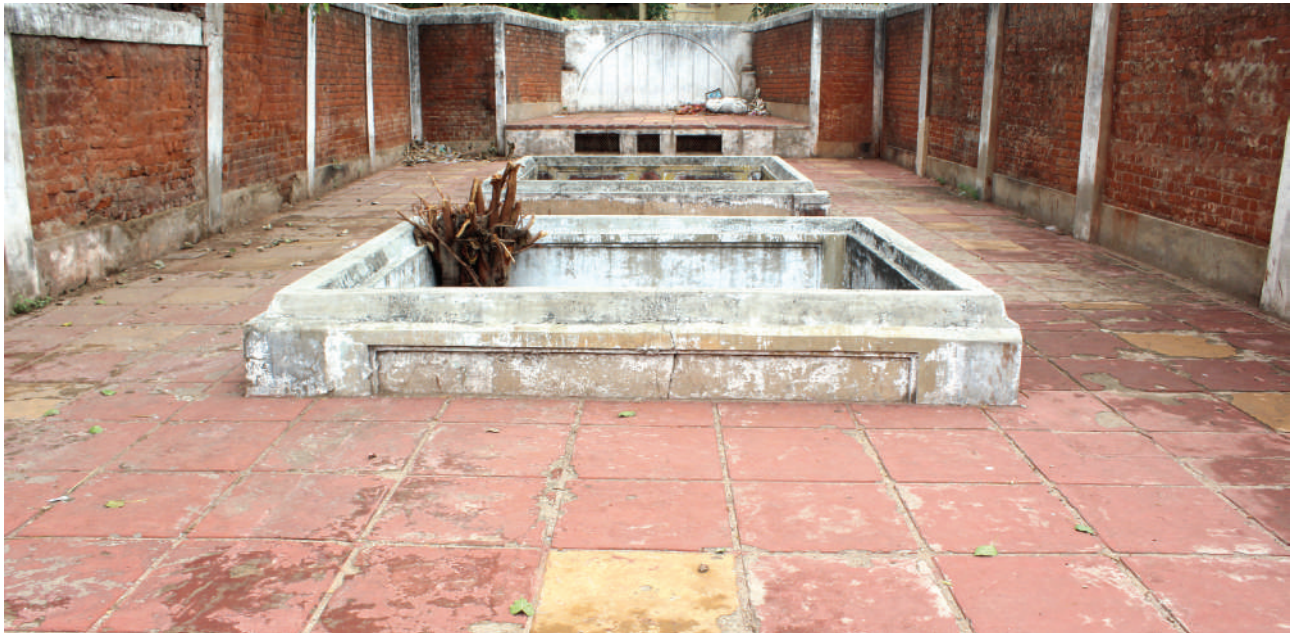
The Vav has been paved over at ground level
