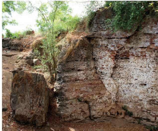
The damage is continuing
