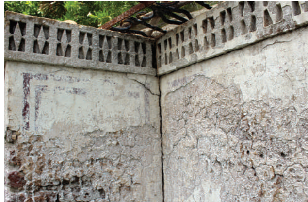
Cracks along the walls.
