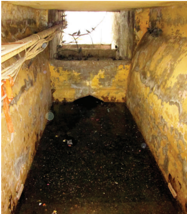
The water inside is putrid
