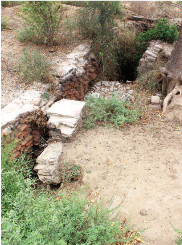
The walls are crumbling
