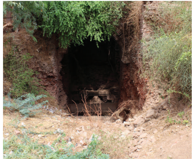
The extent of the damage suggests the stepwell was abandoned long ago
