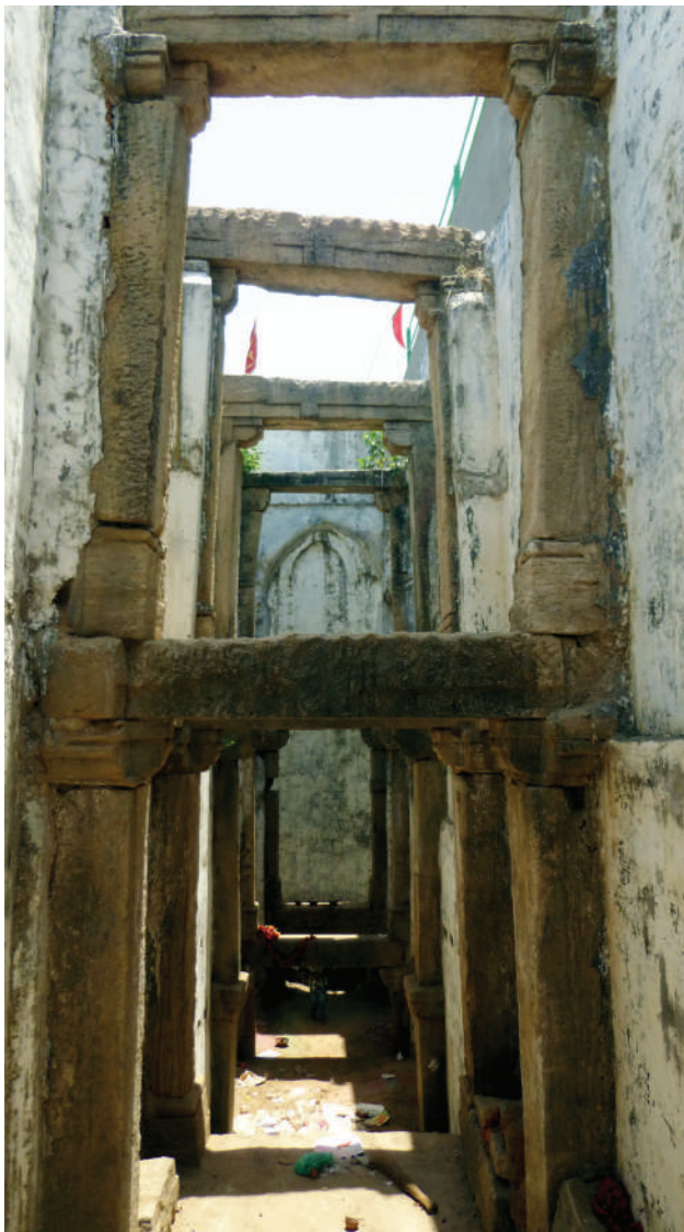
The stepwell is in a state of severe disrepair
