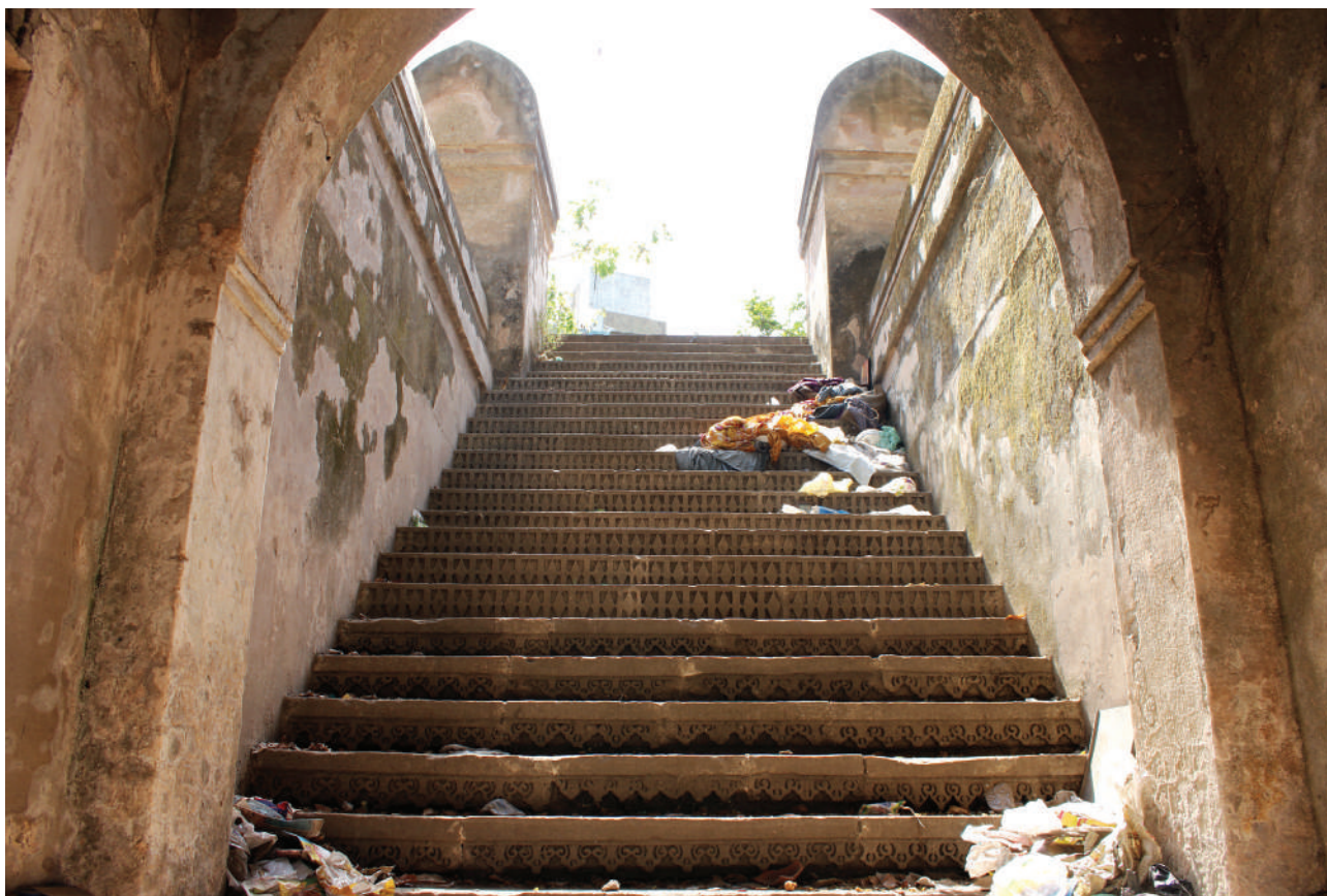
Garbage being dumped inside the well
