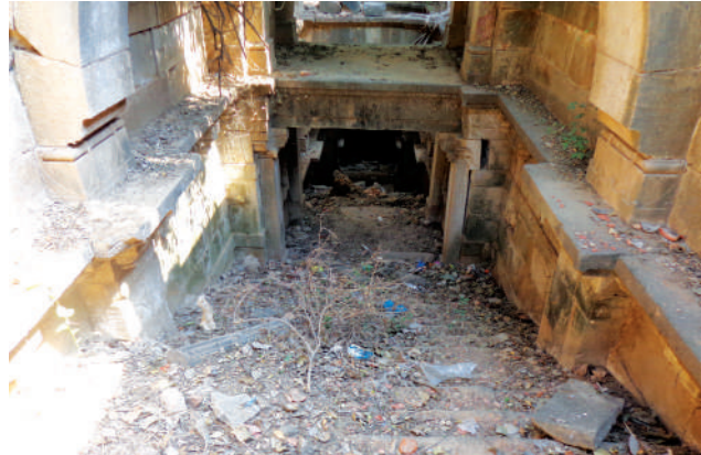
The stepwell is in severe disrepair
