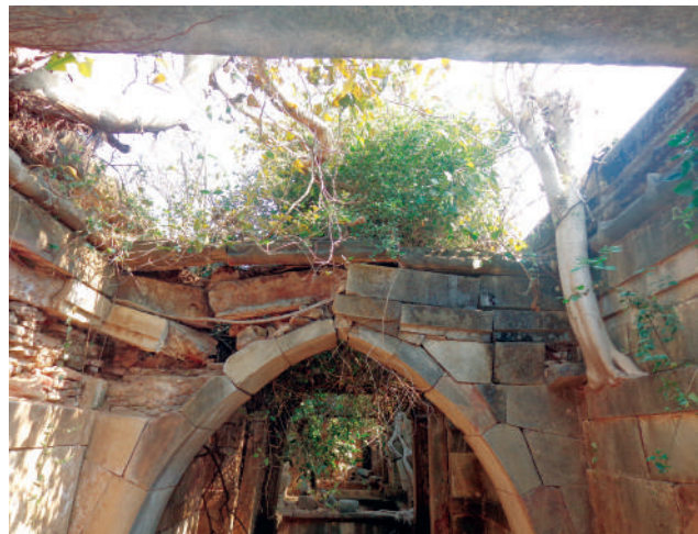
Vegetation is damaging the structure of the stepwell
