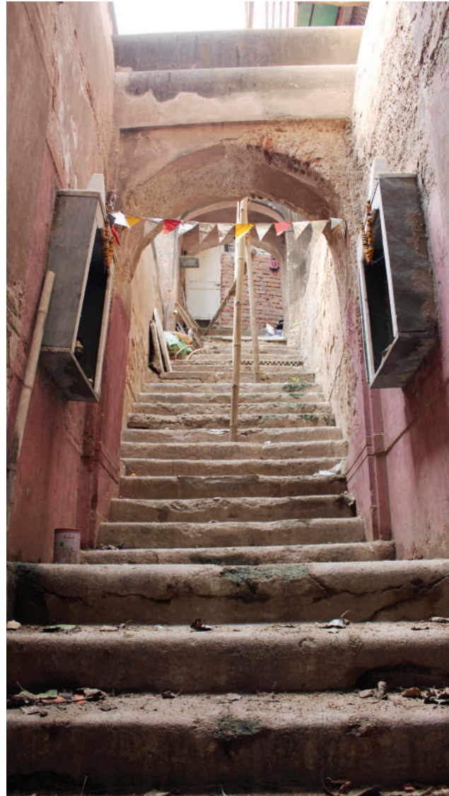
The residents have started encroaching on the structure
