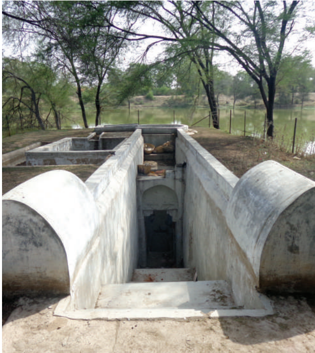
A lot of soil has been filled around the structure
