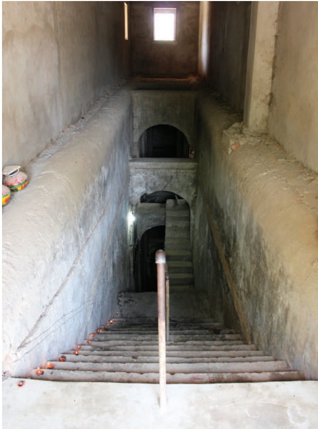
This stepwell is in the process of being encroached on
