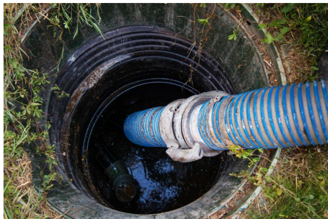
Fig 2.7.3: Left sludge at the bottom
