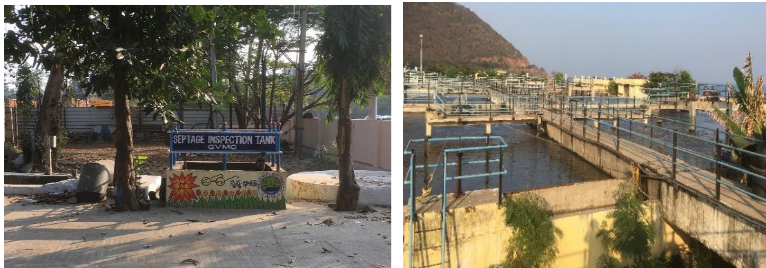
Fig. 4.3.3: Sludge disposal tank connected with STP, Vizag, Andhra Pradesh
