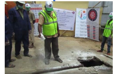
Add chlorine on hose after emptying
