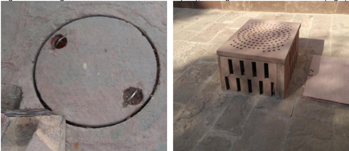
Figure 44 Existing manhole cover at Sardar market (Left), Existing Surface drain near market (Right)
