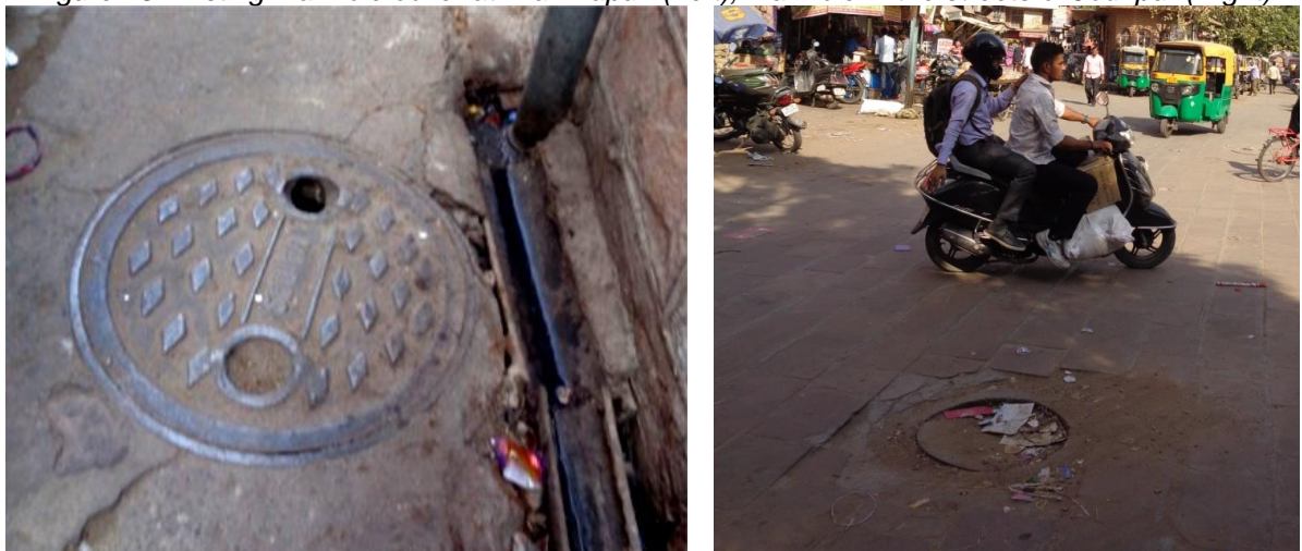
Figure 45 Existing manhole cover at Brahmapuri (Left), Manhole in the streets of Jodhpur (Right)
