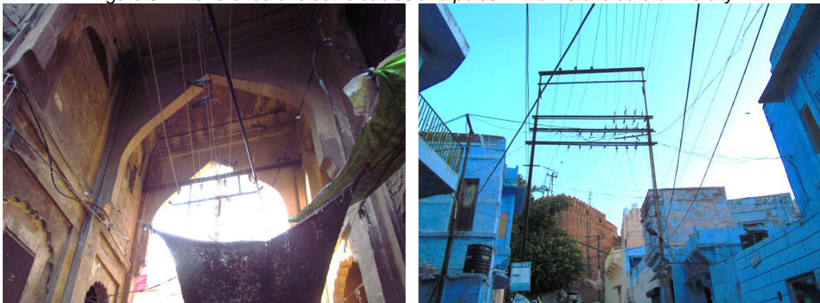
Figure 31 Interference of electric cables and poles in the historic core of the city
