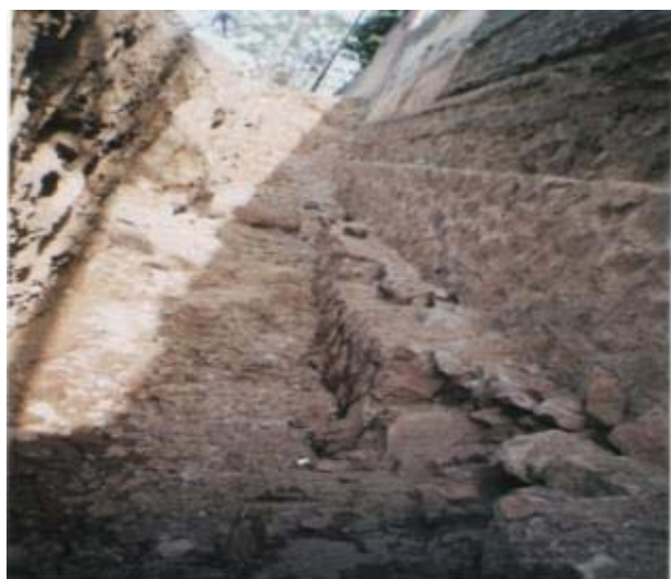
Dilapidated state of water storage tank
