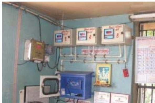
Bulk Flow Meter and Pressure Monitoring Equipments
