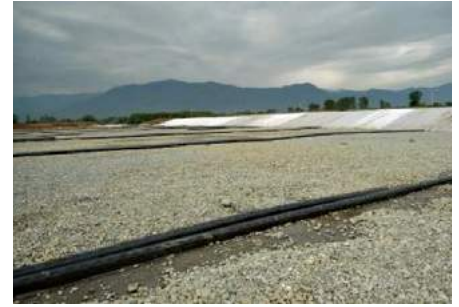
The underground drainage system for leachate collection
