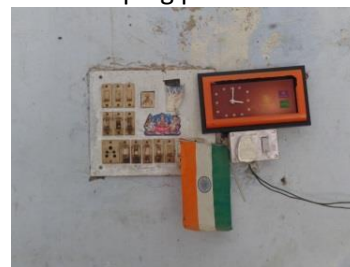
15. Electrical plug points
