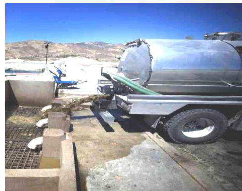
Figure 19 Sludge disposal into inlet chamber of STP
