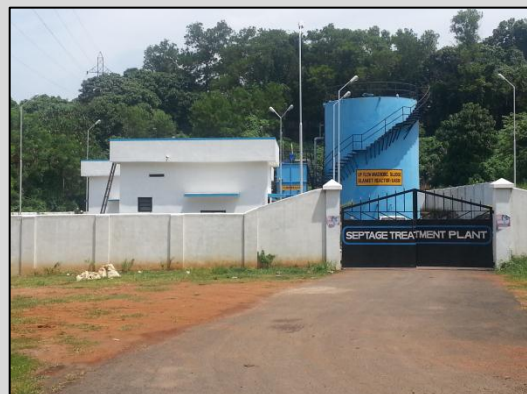
Figure 25 Septage Treatment Plant, Cochin
